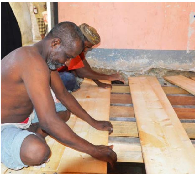
Reconstruction taking place on the Governor's HQ Complex (Former British Residency) main building in Mukalla, Yemen. © Daw'an Architecture Foundation
