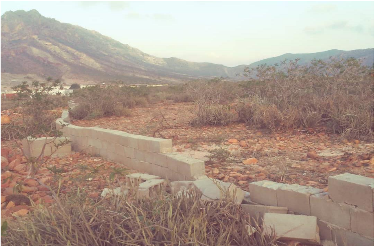
Cyclone damage to the protective wall at rock art site SHP067 in 2022.
